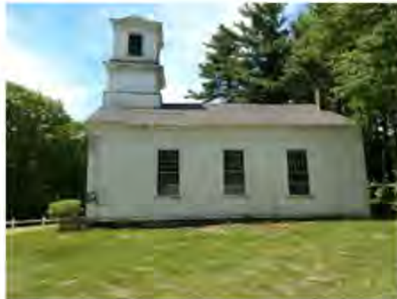
East elevation of church with three large sanctuary windows. Note the leaning-in of the bell tower towards the center of the church. Photo courtesy Steve Bedard.
