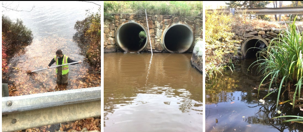
Above: LRPC Staff in the field in Gilmanton evaluating stream crossings, culverts, and CCDS
